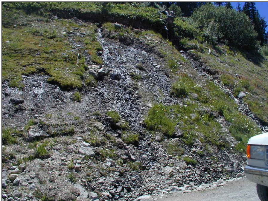
Figure 3. Interception of shallow groundwater on hillslope cut to accommodate a maintenance road contributes to increased flow in ditches and road surfaces (Maholland, 2002).
