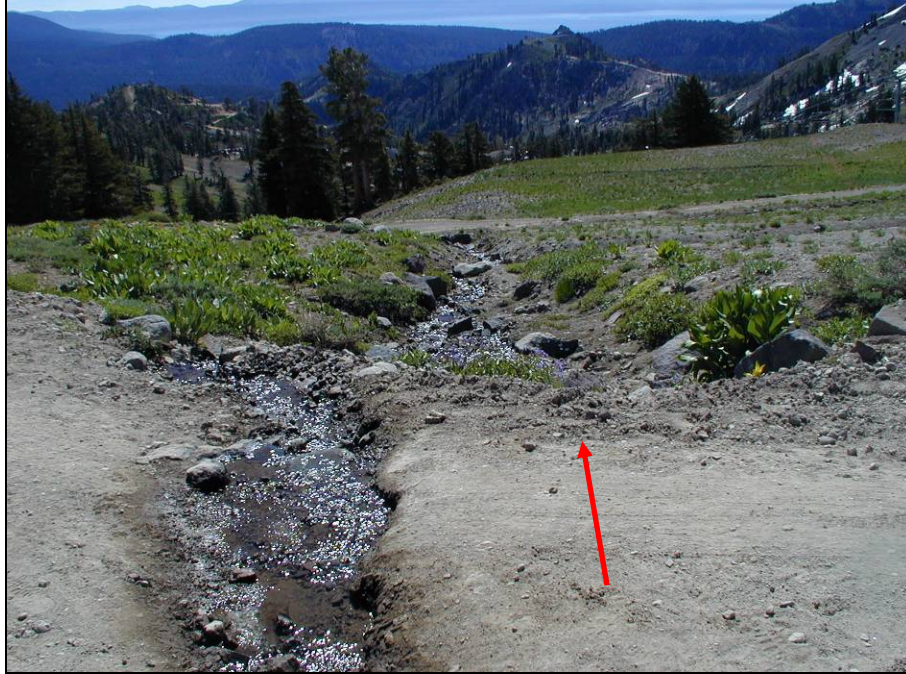
Figure 2. Gully formed on road surface concentrates and directs runoff and sediment to an adjacent stream channel in upper area of the South Fork of Squaw Creek. Red arrow indicates direction of flow (Maholland, 2002).
