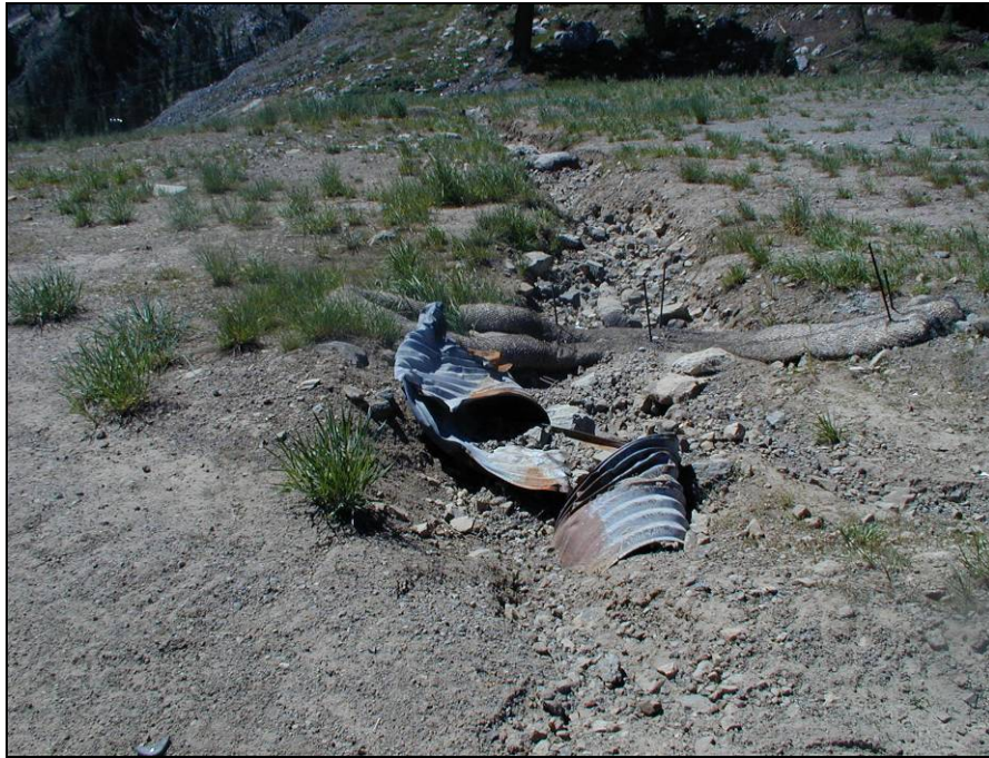
Figure 5. Failed culvert in South Fork subwatershed of Squaw Creek showing evidence of increased sediment and discharge to stream network.
